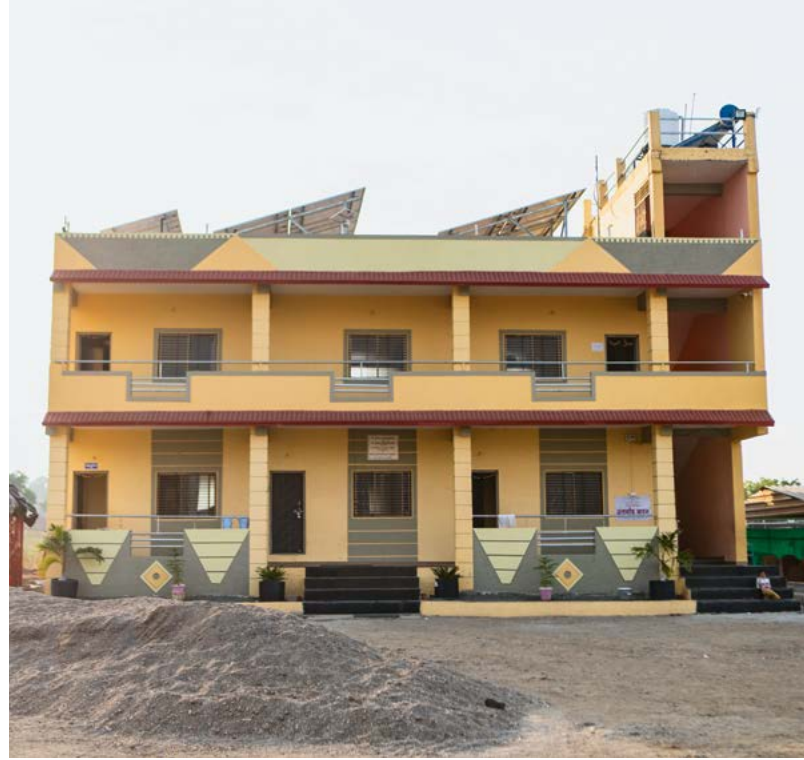
Newly installed solar panels on Balgram Orphanage.
